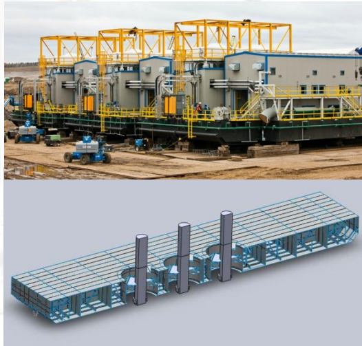
Oil Sands Project: Vibration Response Analysis of Weir Mega Pump Barge
